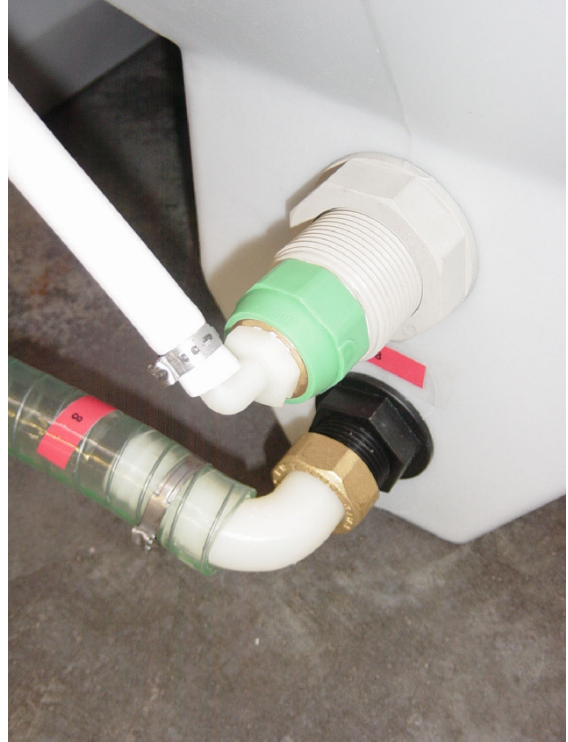
Connection aerator unit
