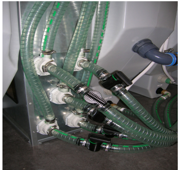
Suction lines + pressure lines
