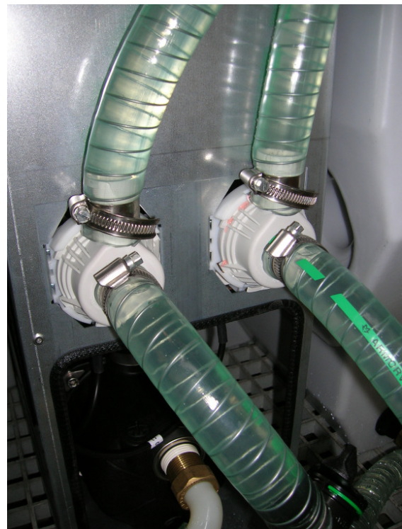
Suction lines + pressure lines
