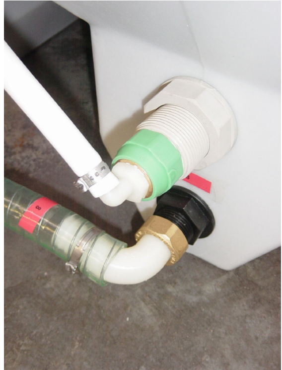
Connection aerator unit
