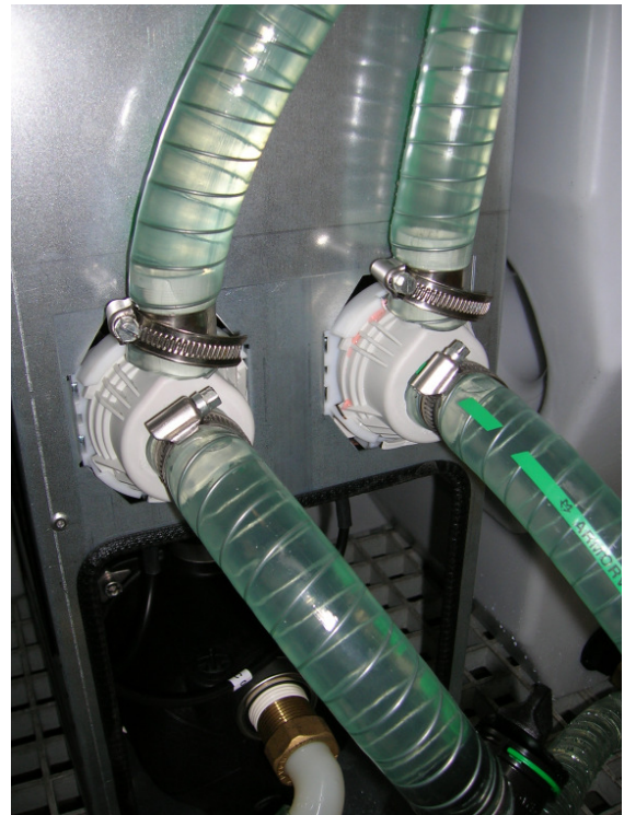
Suction lines + pressure lines
